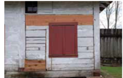
A condition assessment of the exterior walls and frame of this Storehouse at Fort Langley, BC found extensive deterioration of some timbers, which required replacement in kind. The dimensions, hewn finish and species of wood used in the repairs matched those replaced. The photograph shows part of one storehouse wall after the repairs were completed, but before the new timbers were whitewashed.
