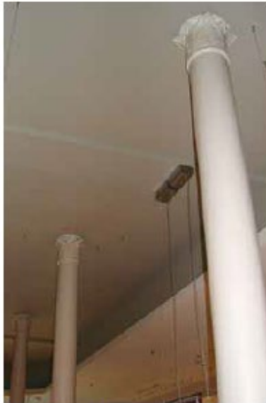
These cast iron columns were uncovered and restored when CentreBeam Place, in St. John, was rehabilitated.
