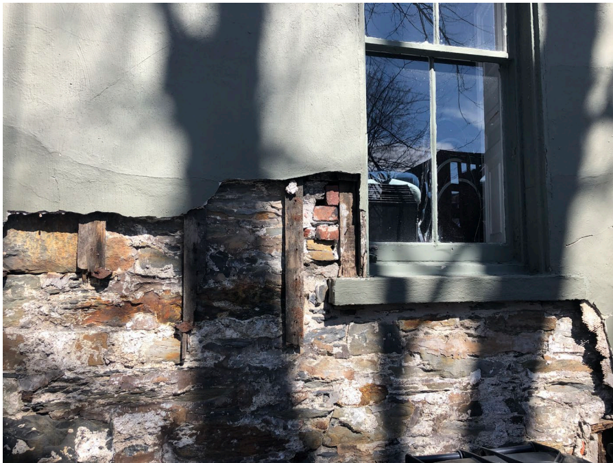
Figure 10: Evidence of original rubble stone walls underneath stucco cladding on south façade (April 9, 2021)
