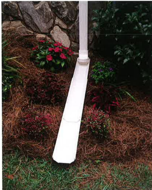
Downspouts should drain the water away from any impervious areas, such as the foundation or driveway, and into vegetated zones.
