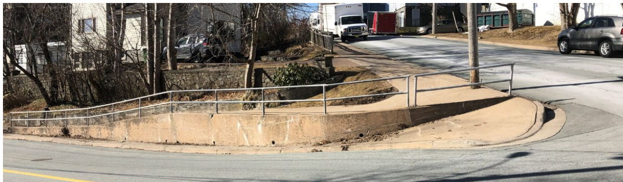
Figure 9: Photo of Accessibility Challenges to be Addressed at Dahlia Crichton Intersection
