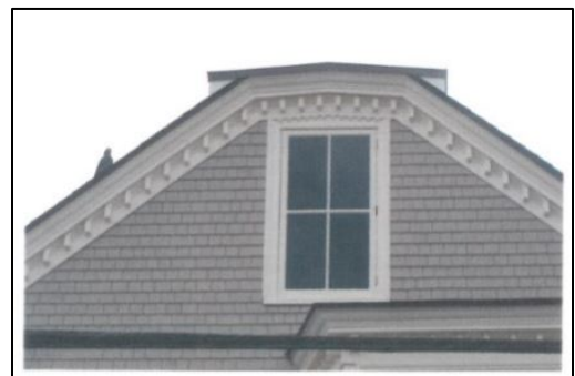
Figure 9: Truncated narrow flat roof with dentils under eave. Source: Heritage Assessment Report – Dr. Allen B. Robertson
