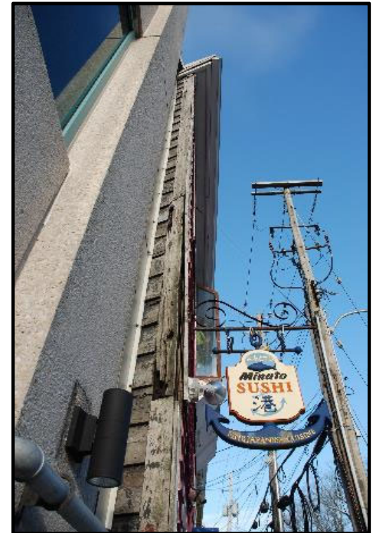
Detail of deteriorated corner board adjacent 5475 Spring Garden Road
