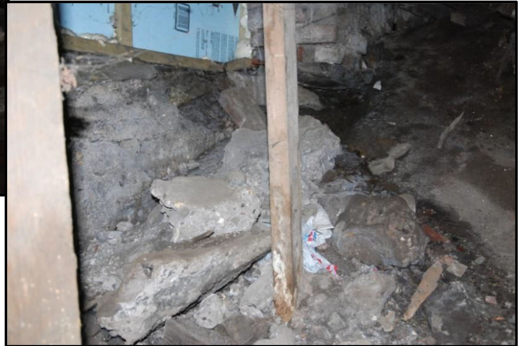
Unsupported foundation wall section
