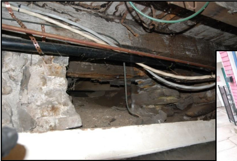
Decayed floor joist at top of foundation wall.
