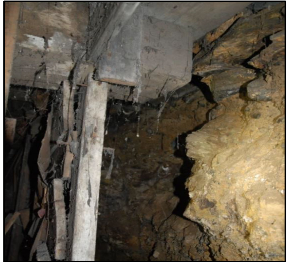
Exposed earth at back of basement
