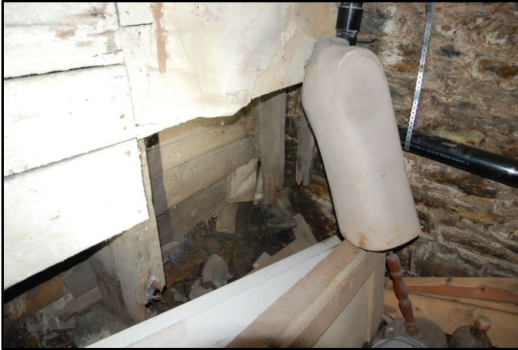
Partition wall at north side of basement rotted and missing framing
