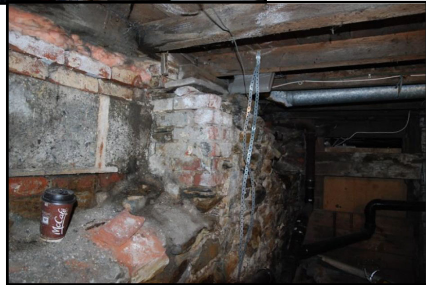
Bulging and deteriorated stone foundation at front. Loose stones and bricks
