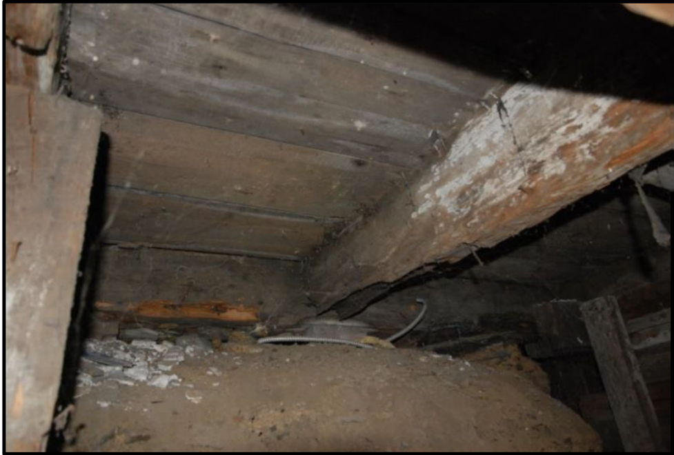
Rotted floor joist and bearing at top of excavated soil face
