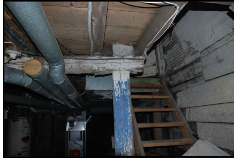
Crushing of bearing at main beam support; note small 4 x 3 floor joists
