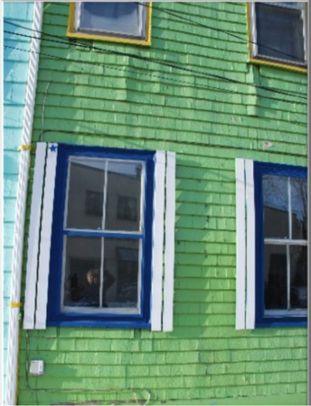
Buckled shingles in front of building
