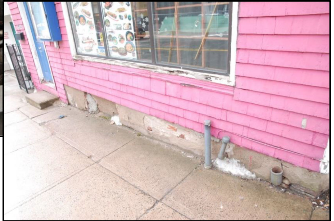
Deteriorated front foundation wall above sidewalk
