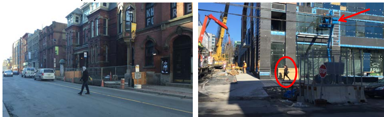
Figure 4 – Without appropriate site controls in place pedestrians are forced to cross streets at unsafe locations or pass directly through an unprotected work area and even underneath active equipment.
