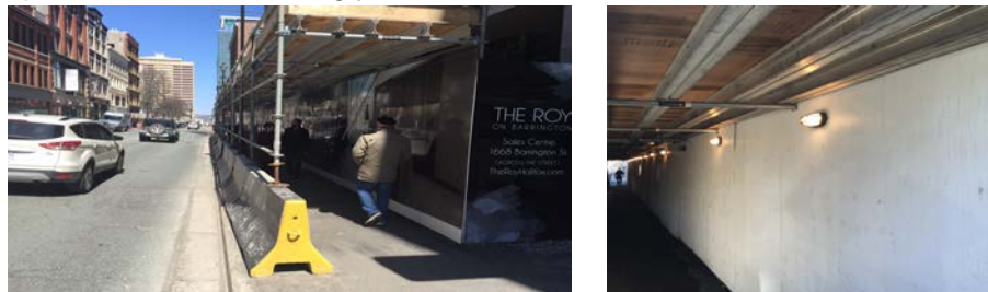
Figure 5 – Solid construction hoarding provides pedestrian protection from vehicles, overhead objects, and provides physical separation from the site activities. Lighting for covered ways is an important consideration.
