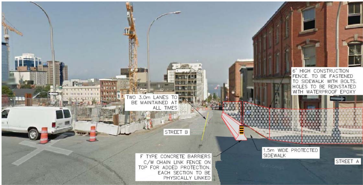
Figure 2 – Proposed protected walkway; Street B. Due to the active construction site on opposite side of Street B, therefore there is no sidewalk on the other side of the street to which direct pedestrians.
