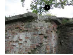
FRONT WALL - CONCRETE CAP TO BE REFORMED
