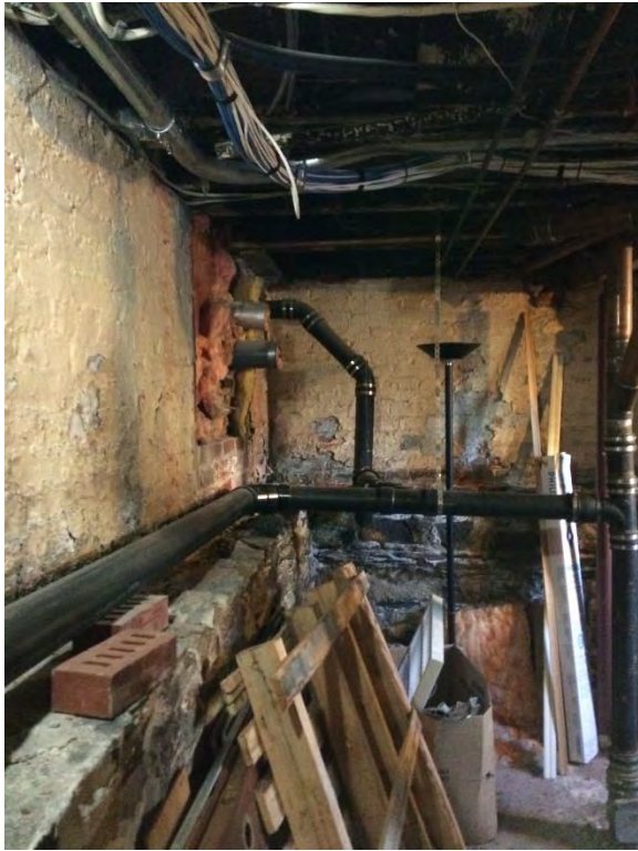
Existing Step and Transition in Foundation Wall Between Stone and Brick in rear L.
