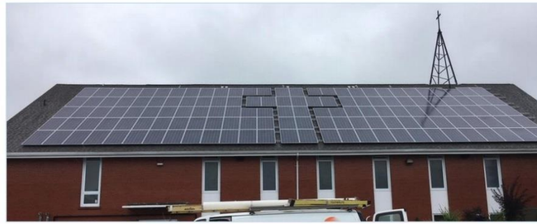
Figure 1: Completed solar electric installation at the Woodlawn United Church in Dartmouth
