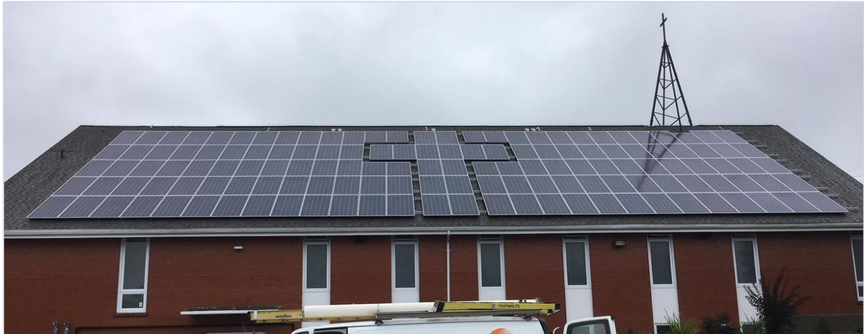
Figure 1: Completed solar electric installation at the Woodlawn United Church in Dartmouth
