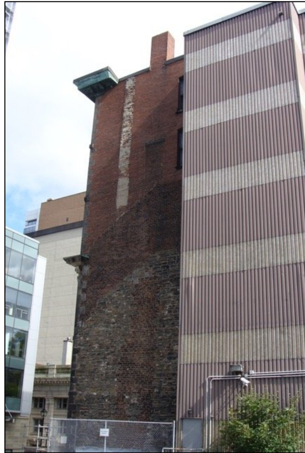
Figure 11: An enclosed fire escape with corrugated metal siding does not cover up character-defining elements, however, nor does it complement the building's character.
