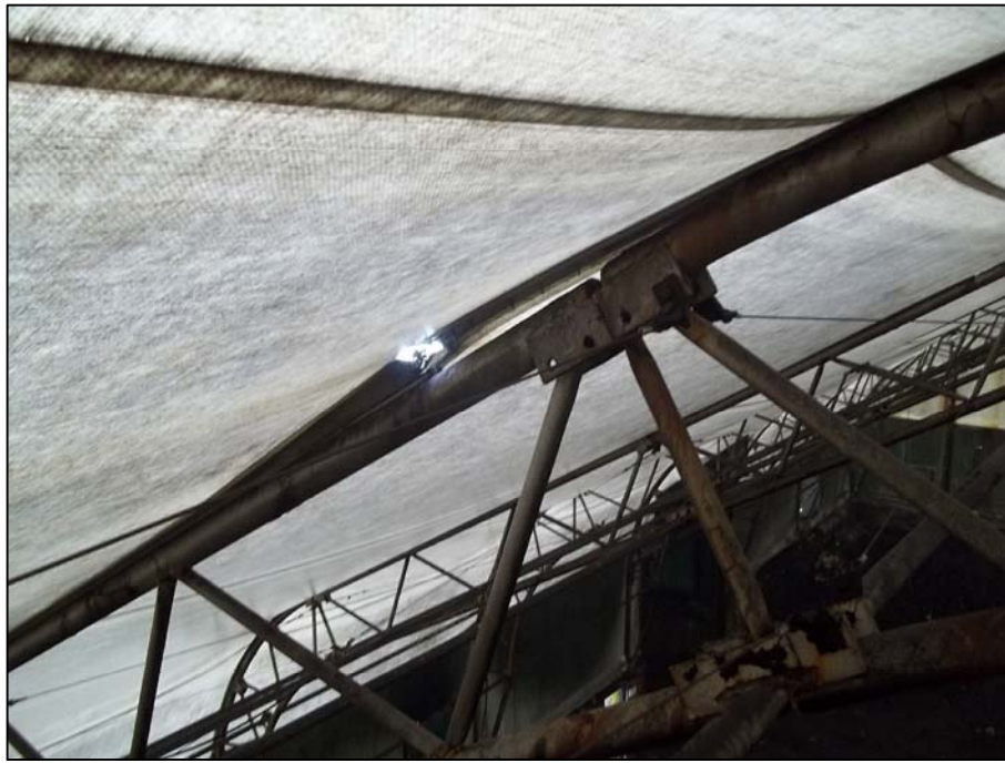
PHOTO 23 - TYPICAL TEAR IN ROOF FABRIC NEAR TRUSS
