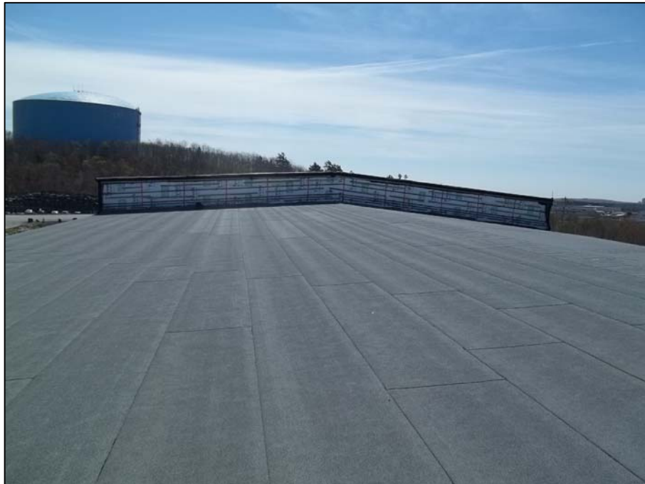
PHOTO 22 - WALL AT JUNCTION OF HIGH ROOF AND LOW ROOF WITH ONLY TYVEK AIR BARRIER
