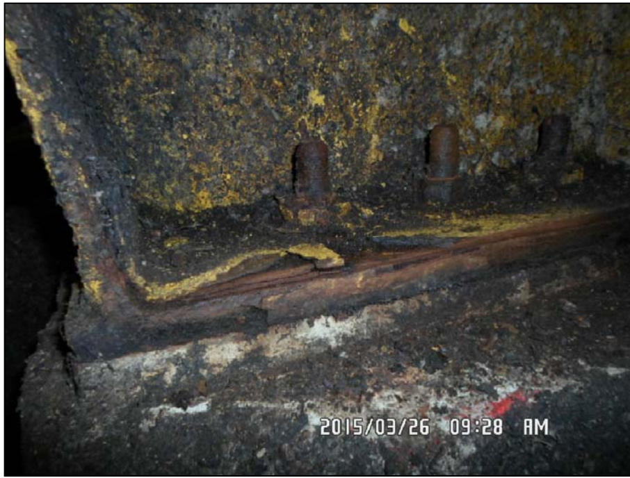
PHOTO 11 - RECEIVING BUILDING-BASE PLATE AND ANCHOR ROD CORROSION AND STEEL DELAMINATION AT GRIDLINE H1
