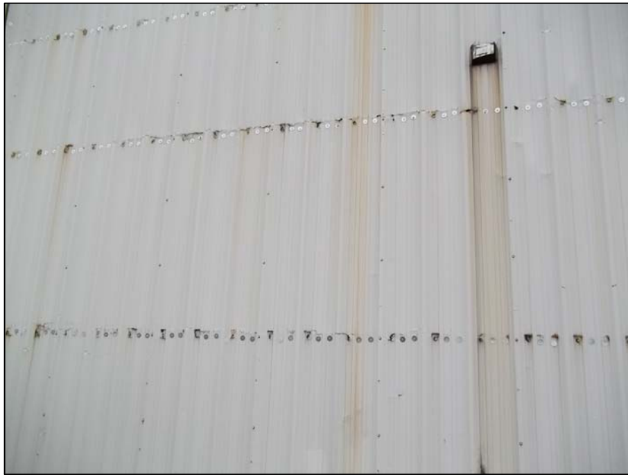
PHOTO 7 - AREA ALONG EAST ELEVATION WHERE SIDING HAS COMPLETELY CORRODED IN AREAS ADJACENT TO WALL GIRTS AND HAS BEEN PINNED
