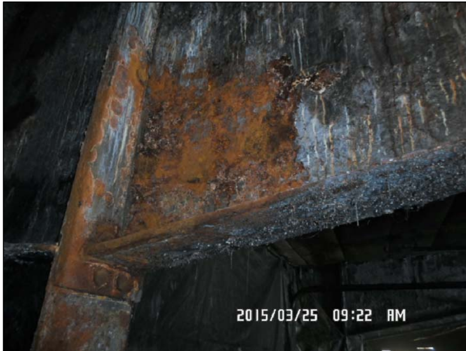
PHOTO 16 - VESSEL AREA-TYPICAL FAILURE OF EPOXY PAINT SYSTEM AND ASSOCIATED SURFACE CORROSION
