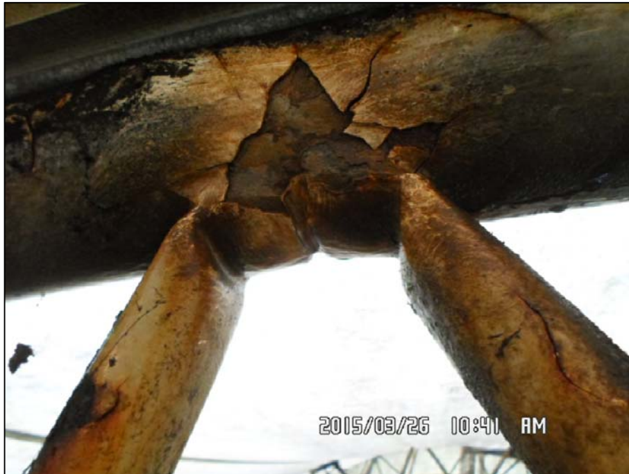
PHOTO 28 - SCREENING BUILDING-EPOXY PAINT CRACKED AND FLAKED OFF EXPOSING GALVANIZED STEEL WITH LOCALIZED AREAS OF CORROSION
