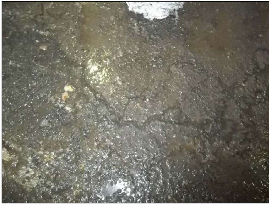
PHOTO 5 - TYPICAL CRACKING AND DAMAGE TO CONCRETE FLOOR IN RECEIVING AREA
