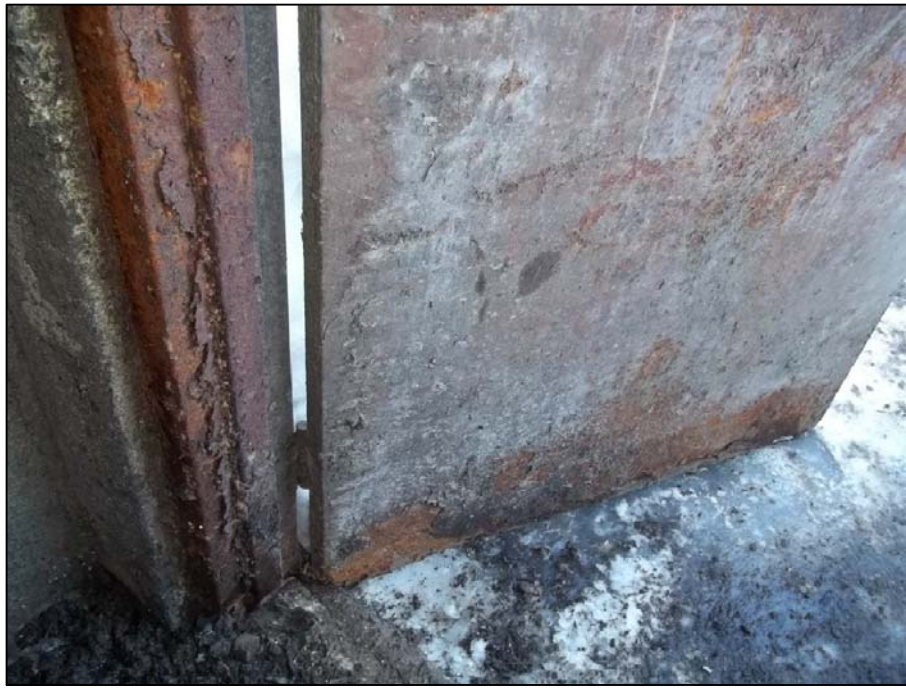
PHOTO 7 - CORROSION DAMAGE TO DOOR AND FRAME NEAR SPRINKLER ROOM IN VESSEL AREA
