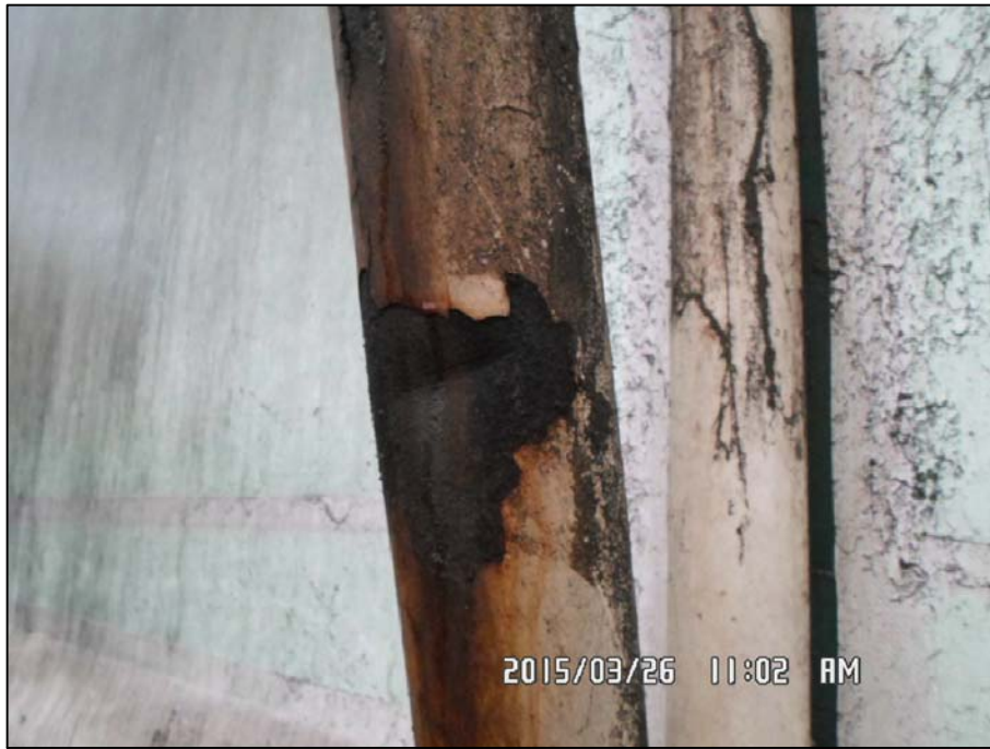
PHOTO 27 - SCREENING BUILDING-DAMAGE TO BOTTOM CHORD OF 6TH TRUSS FROM NORTH AT WEST END NEAR THE SUPPORT
