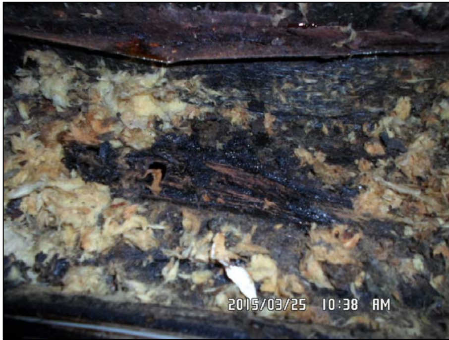
PHOTO 15 - VESSEL AREA-SOUTH WALL GIRTS NEAR FLOOR EXHIBITING SURFACE CORROSION AND SECTION LOSS
