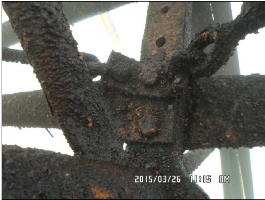
PHOTO 19 - CURING BUILDING-TYPICAL ORGANIC MATERIAL ACCUMULATION
