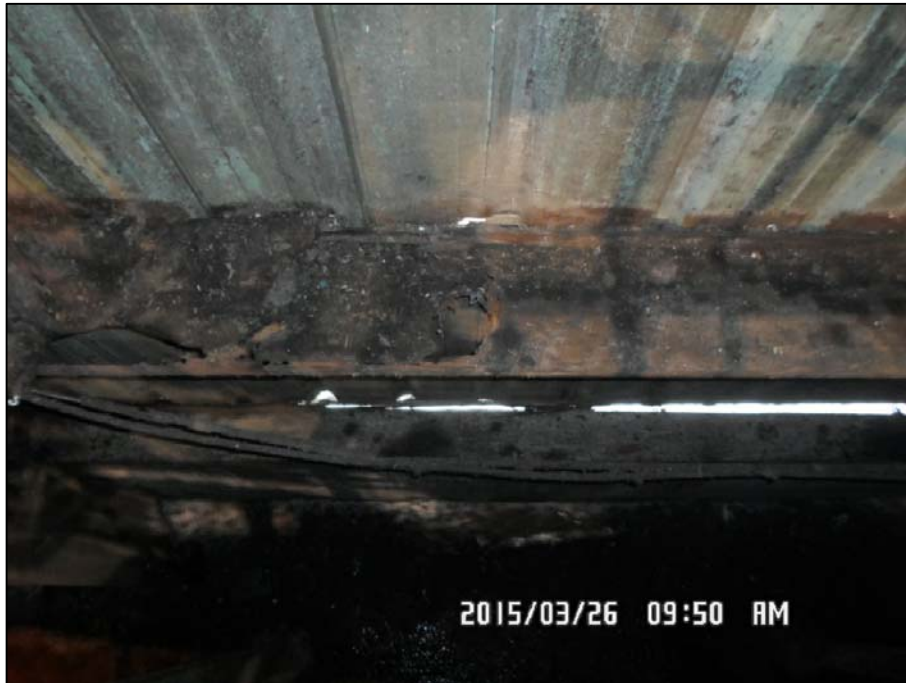
PHOTO 12 - RECEIVING BUILDING-GIRT CORROSION DAMAGE AND LOSS OF SECTION
