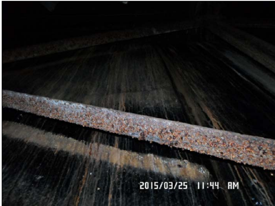
PHOTO 18 - CURING AREA-TYPICAL SURFACE CORROSION ON TRUSSES
