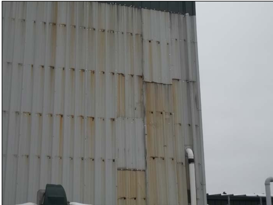
PHOTO 8 - AREA IN SOUTHWEST CORNER WHERE SIDING HAD PREVIOUSLY BLOWN OFF AND HAS BEEN TEMPORARILY PUT BACK IN PLACE USING PINS
