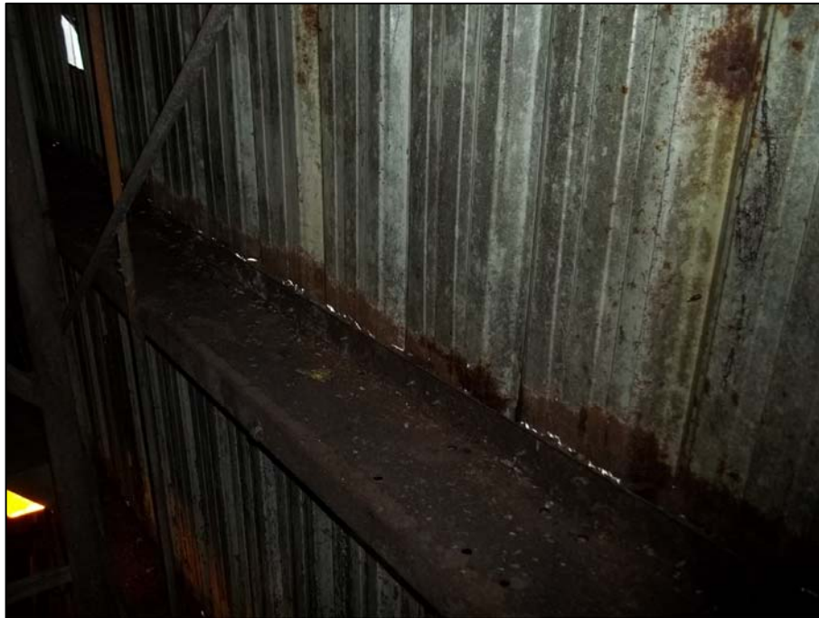
PHOTO 10 - TYPICAL CORROSION OF METAL SIDING IN AREAS ADJACENT TO WALL GIRTS
