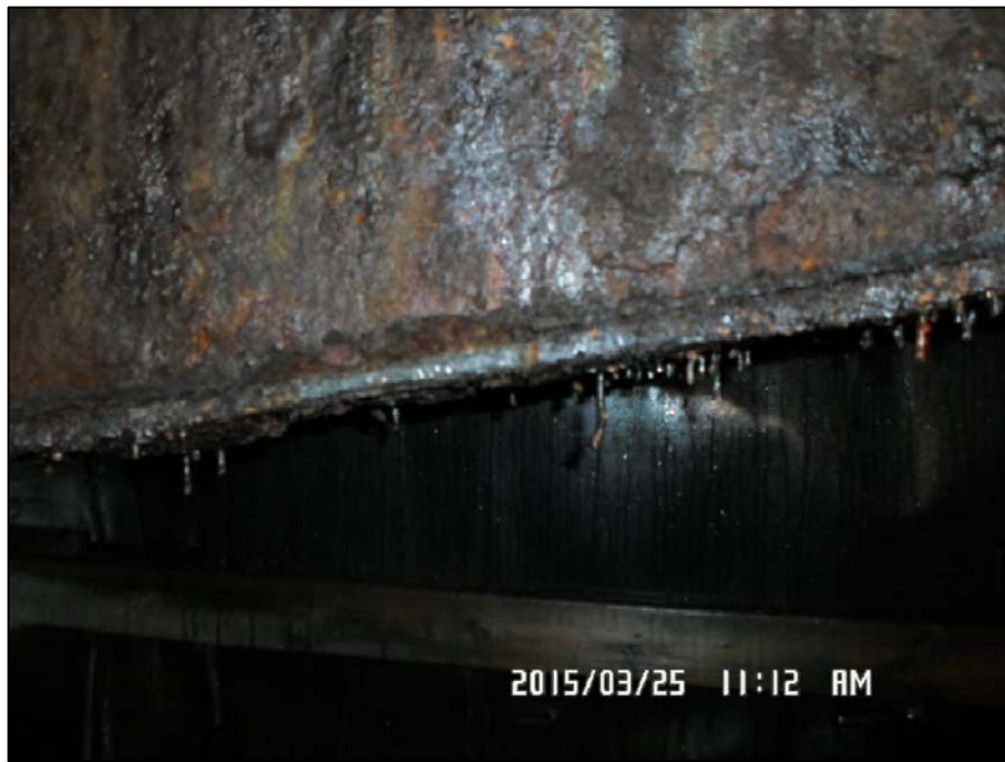
PHOTO 17 - VESSEL AREA-TYPICAL ACCUMULATION OF ORGANIC MATERIAL ON MAIN FRAME
