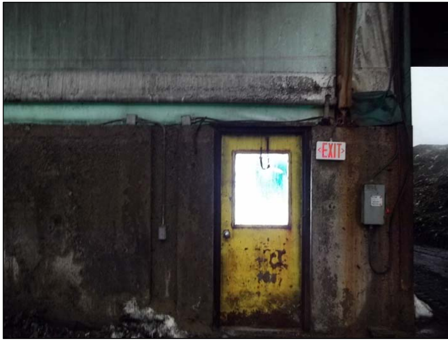
PHOTO 25 - TYPICAL CORROSION OF MAN DOORS AND FRAMES IN SCREENING BUILDING
