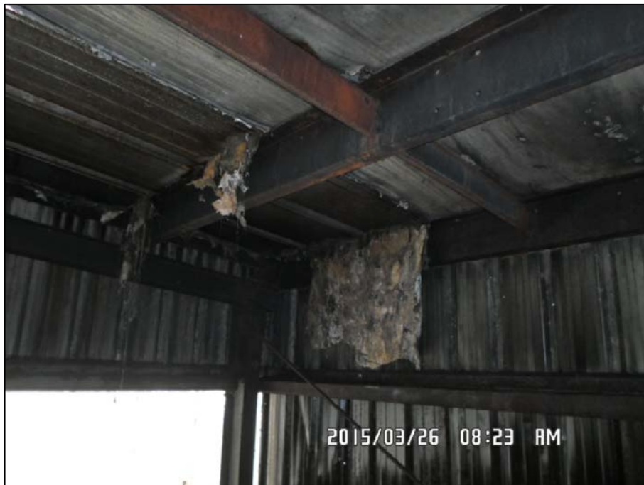
PHOTO 14 - RECEIVING BUILDING - TYPICAL ROOF INSULATION DAMAGE DUE TO PREVIOUS RODENT PROBLEMS
