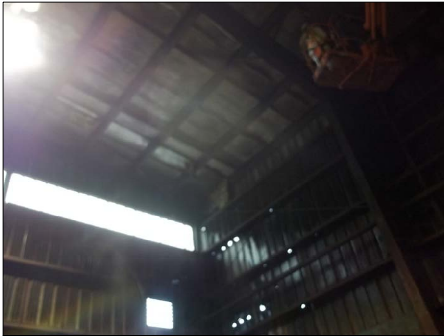
PHOTO 9 - INTERIOR OF SOUTHWEST CORNER WHERE METAL SIDING THAT PREVIOUSLY BLEW OFF HAS BEEN TEMPORARILY PUT BACK IN PLACE WITH PINS
