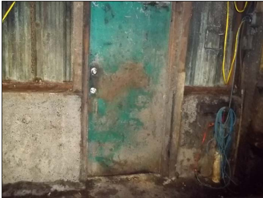
PHOTO 6 - CORROSION OF METAL MAN DOOR AND FRAME IN RECEIVING BUILDING
