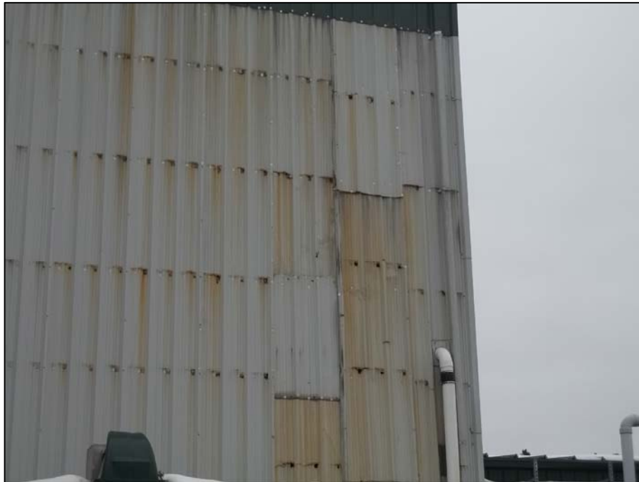
PHOTO 8 - AREA IN SOUTHWEST CORNER WHERE SIDING HAD PREVIOUSLY BLOWN OFF AND HAS BEEN TEMPORARILY PUT BACK IN PLACE USING PINS
