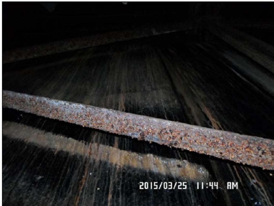
PHOTO 18 - CURING AREA-TYPICAL SURFACE CORROSION ON TRUSSES
