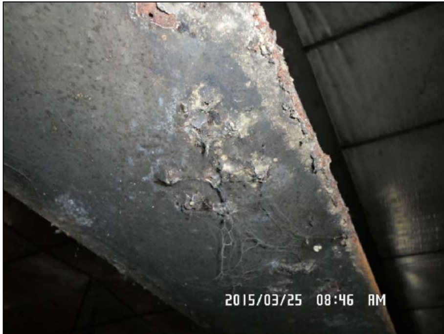
PHOTO 12 - RECEIVING AREA-LOCALIZED AREAS OF CORROSION ON BOTTOM FLANGE OF MAIN FRAMES
