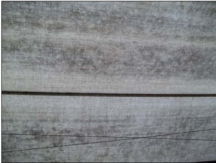
PHOTO 21 - TYPICAL CONDITION OF SCREENING BUILDING FABRIC COVERING
