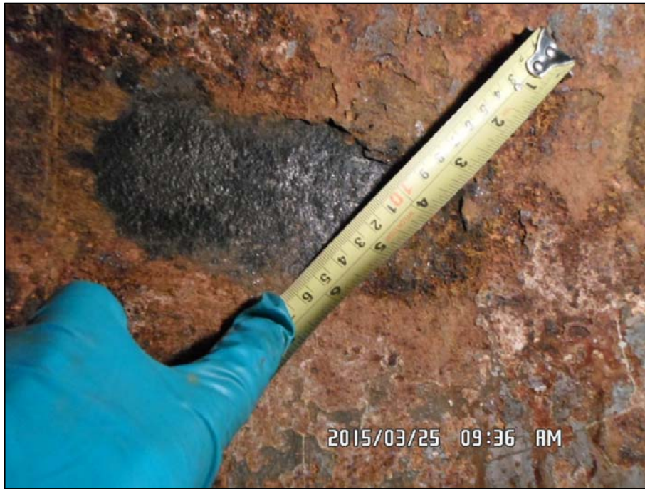
PHOTO 13 - VESSEL AREA-FAILED EPOXY PAINT SYSTEM AND ROUGHENED SURFACE INDICATIVE OF SURFACE CORROSION
