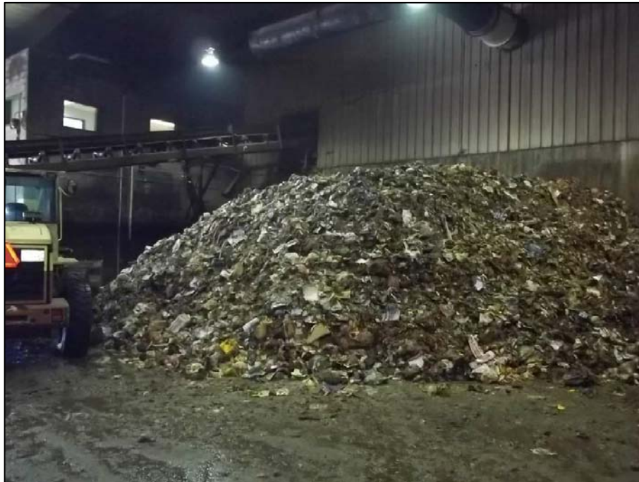
PHOTO 6 - WATER PONDING ON FLOOR OF RECEIVING AREA DUE TO DAMAGED CONCRETE SLAB
