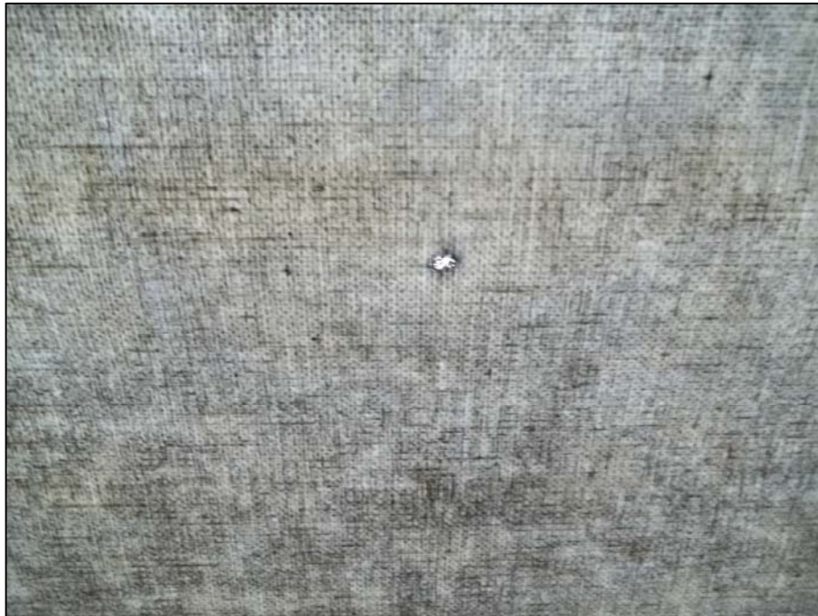
PHOTO 24 - HOLE IN FABRIC ROOF COVERING OF SCREENING BUILDING
