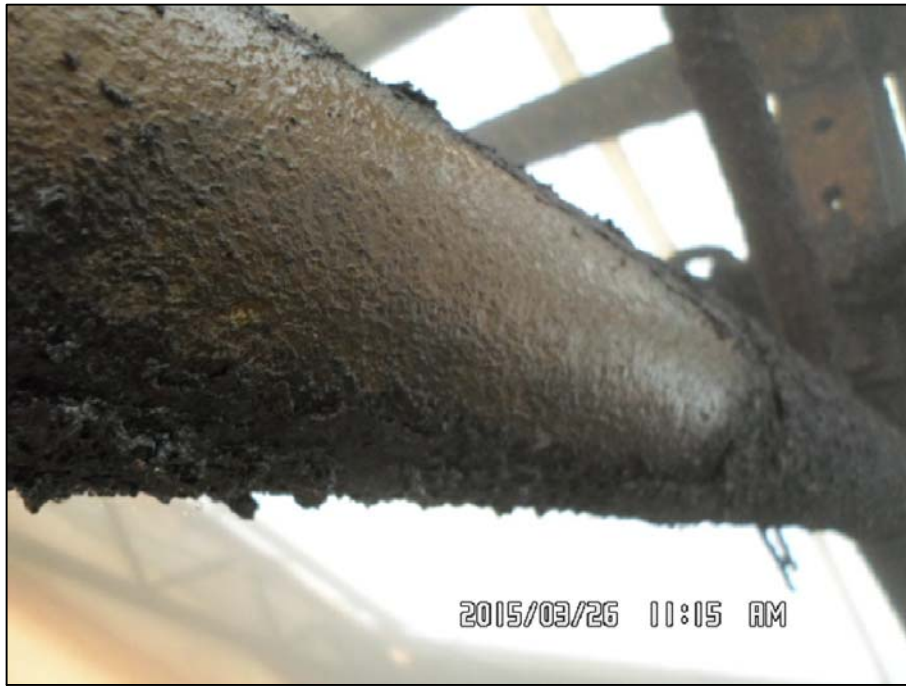
PHOTO 17 - CURING BUILDING-ROUGHENED SURFACE INDICATIVE OF SURFACE CORROSION EXPOSED BENEATH ACCUMULATED ORGANIC MATERIAL
