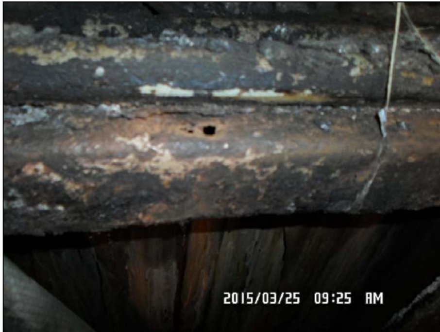
PHOTO 14 - VESSEL AREA-SOUTH WALL GIRTS NEAR EAVE EXHIBITING CORROSION AND SECTION LOSS
