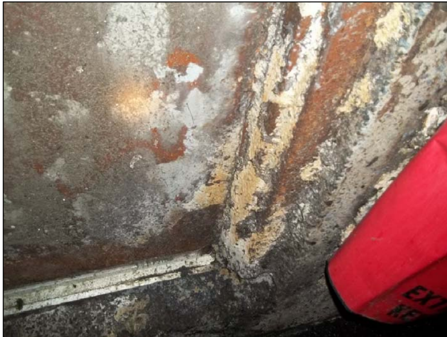
PHOTO 8 - CORROSION TO MAN DOOR AND FRAME ALONG SOUTH ELEVATION OF VESSEL AREA
