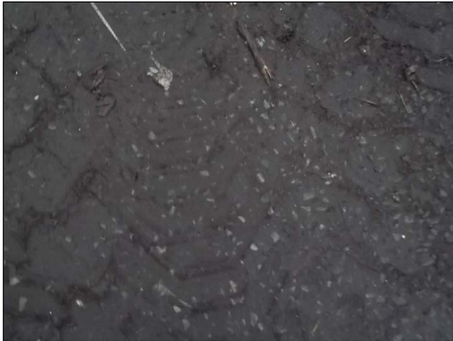
PHOTO 26 - TYPICAL CONDITION OF CONCRETE FLOOR IN AREA ADJACENT TO SCREENING EQUIPMENT
