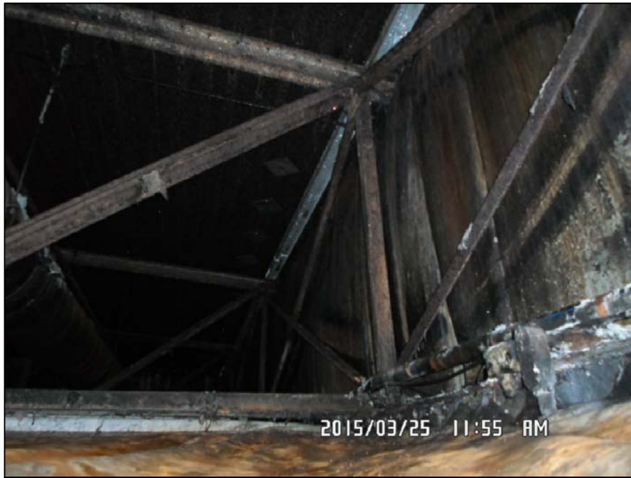
PHOTO 19 - CURING AREA-SURFACE CORROSION ON TRUSSES
