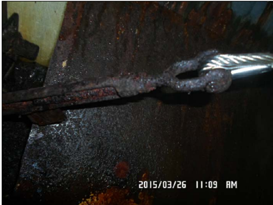
PHOTO 18 - CURING BUILDING-TYPICAL CORROSION ON TURNBUCKLE
