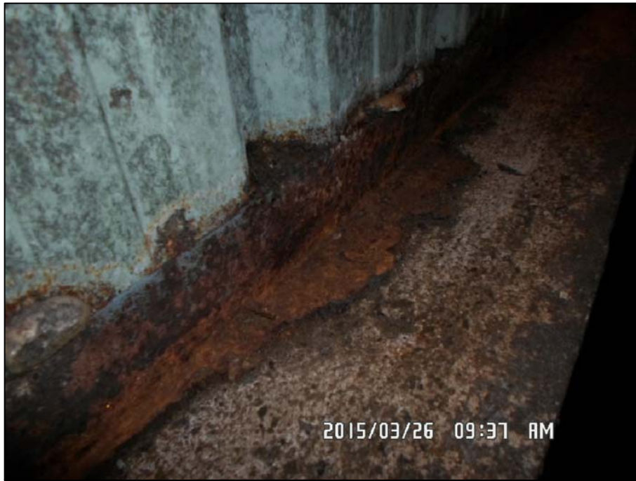
PHOTO 15 - RECEIVING BUILDING-TYPICAL BASE ANGLE CORROSION AND LOSS OF SECTION
