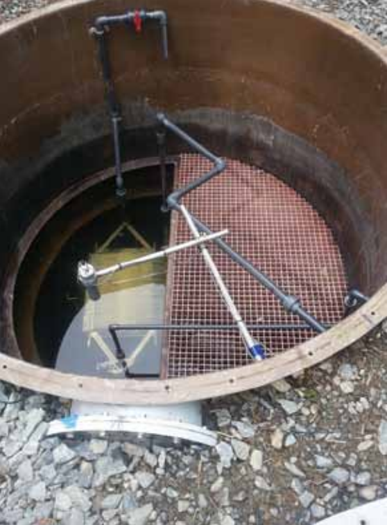
Frame WWTF producing high quality effluent
