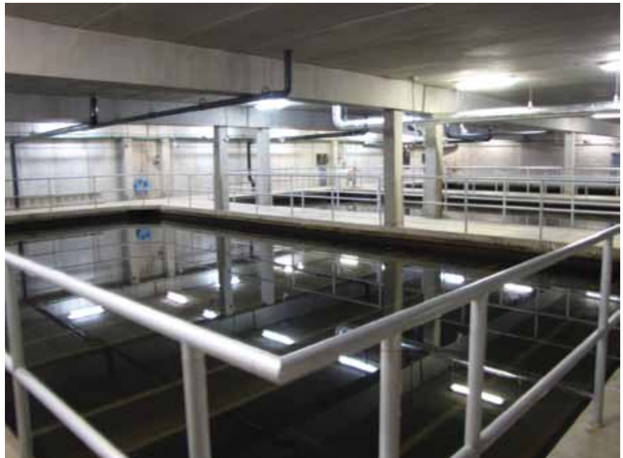
Pockwock water treatment facility, filter gallery
