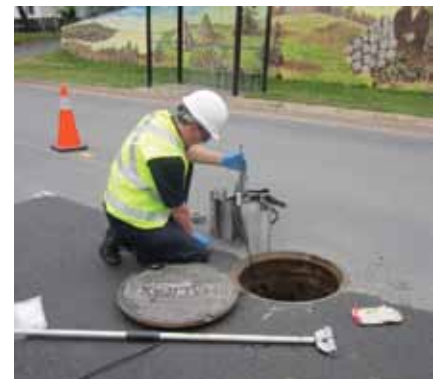
Environmental Engineering staff install a flow meter to monitor stormwater discharge to the wastewater system.
