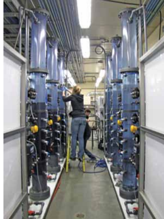
Continuous research at the Pockwock Pilot plant
