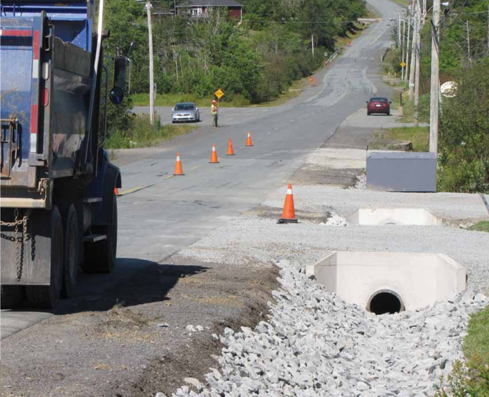
Investing in culvert and ditch infrastructure to improve stormwater service on Pockwock Road
