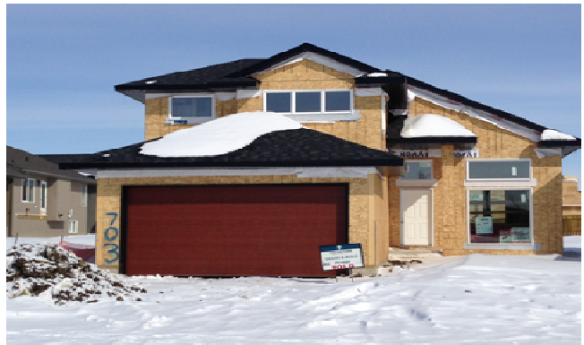
A secondary suite is being constructed in this new home in the Stonebridge neighbourhood.
