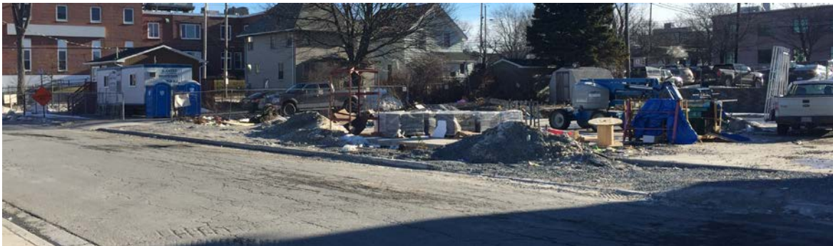
Figure 1 – Construction debris on unprotected sidewalks and streets.
