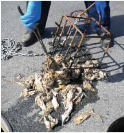
Environmental Engineering staff removing rags, wipes and debris from the wastewater system
