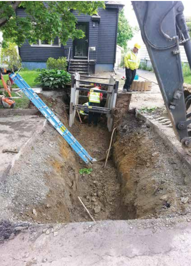
Left: Good trench; Right: Bad trench, an accident waiting to happen
