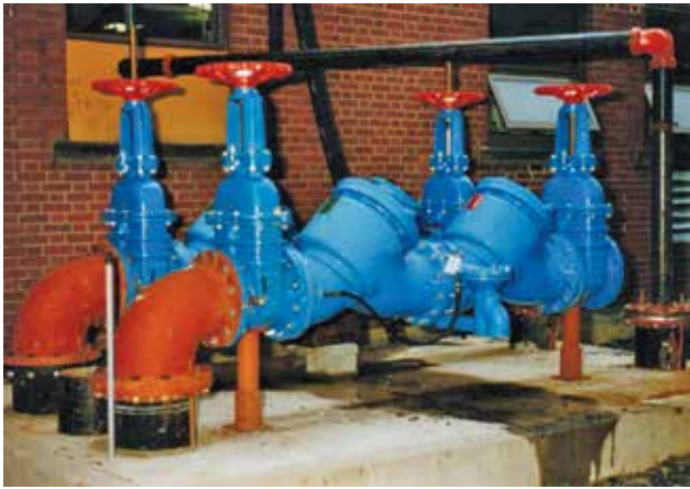
Backflow prevention devices to prevent cross contamination
