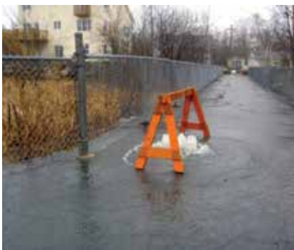
The result of excess stormwater in the wastewater system – a system surcharging
