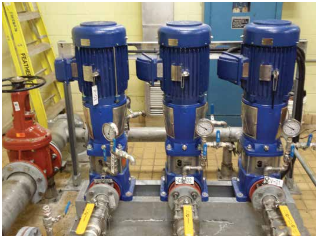
New High Efficiency Pumps and Motors Installed at Highway No. 7 Water Booster Station
