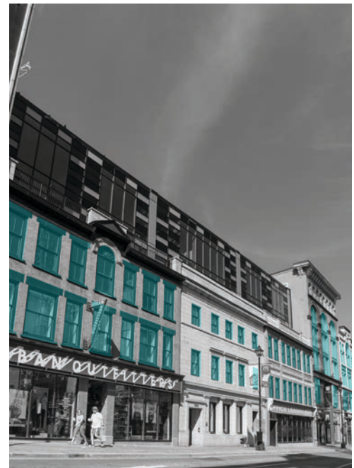
Figure 59. Historic lintels and the original fenestration pattern has been retained in this redevelopment project.
