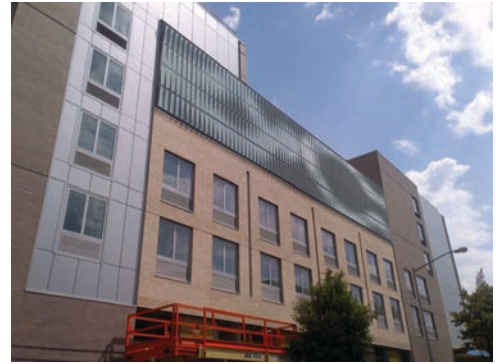
Figure 51. Mechanical equipment and utilities are screened from the public realm using an aluminum and glass wall
