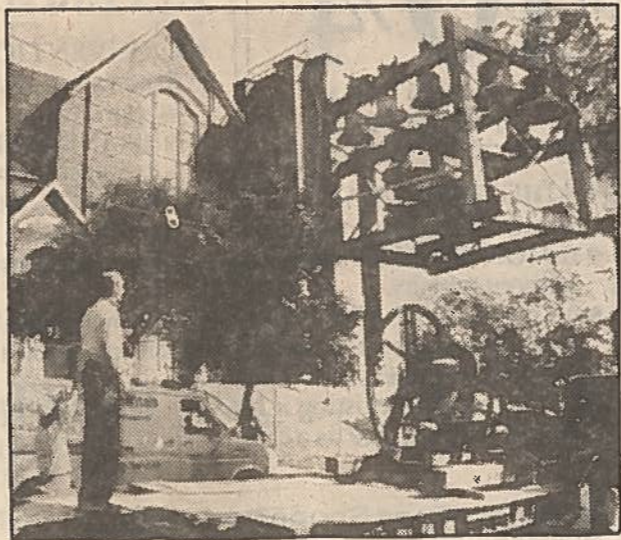
Bells are removed from United Memorial Church for storage pending installation in the memorial tower.
