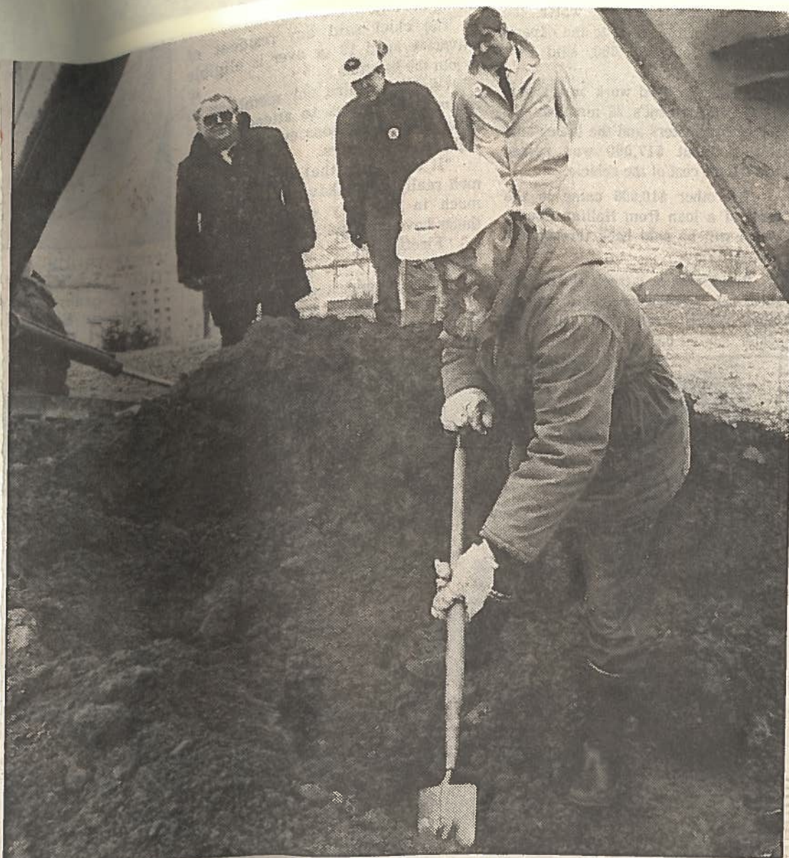
CAREFUL WORK — Engineers and archaeologists will keep a close watch for historic artifacts and clues to the exact location of the original Fort Needham as construction of the Halifax Explosion Memorial Bells monument proceeds. During preliminary soil testing, city historian Lou Collins closely inspects piles of topsoil along with Frank Harrington, memorial bells committee; Bill Sutherland, Jacques Whitford and Associates, and John Dow, Whitman Benn and Associates. Wamboldt-Waterfield
