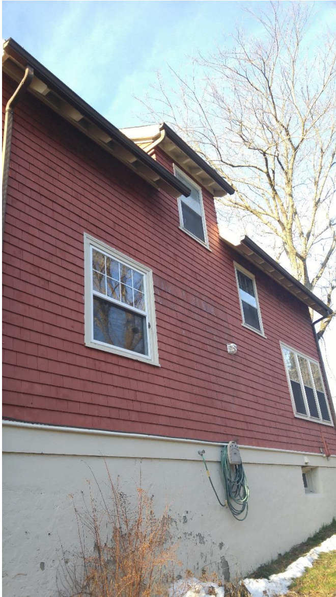
Figure 3: East elevation showing shed dormer, eight-over-one hung windows, wooden shingles, and exposed rafters beneath overhanging eaves
