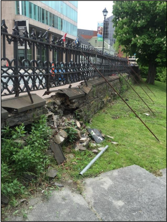
Figure 11: Failed wall section on Argyle Street.
