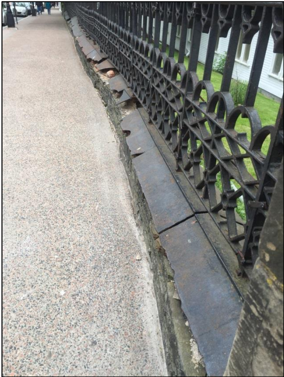
Figure 12: Bowed wall section & broken metal wall cap.
