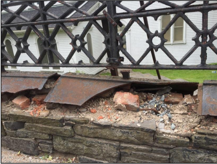
Figure 13: Failed metal cap and brick top course.
