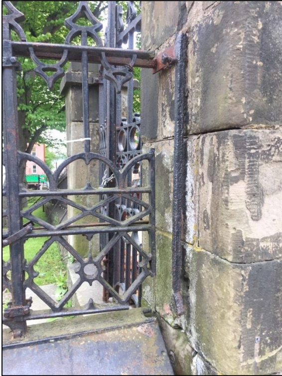
Figure 10: Ironwork failing at the Prince Street gates.
